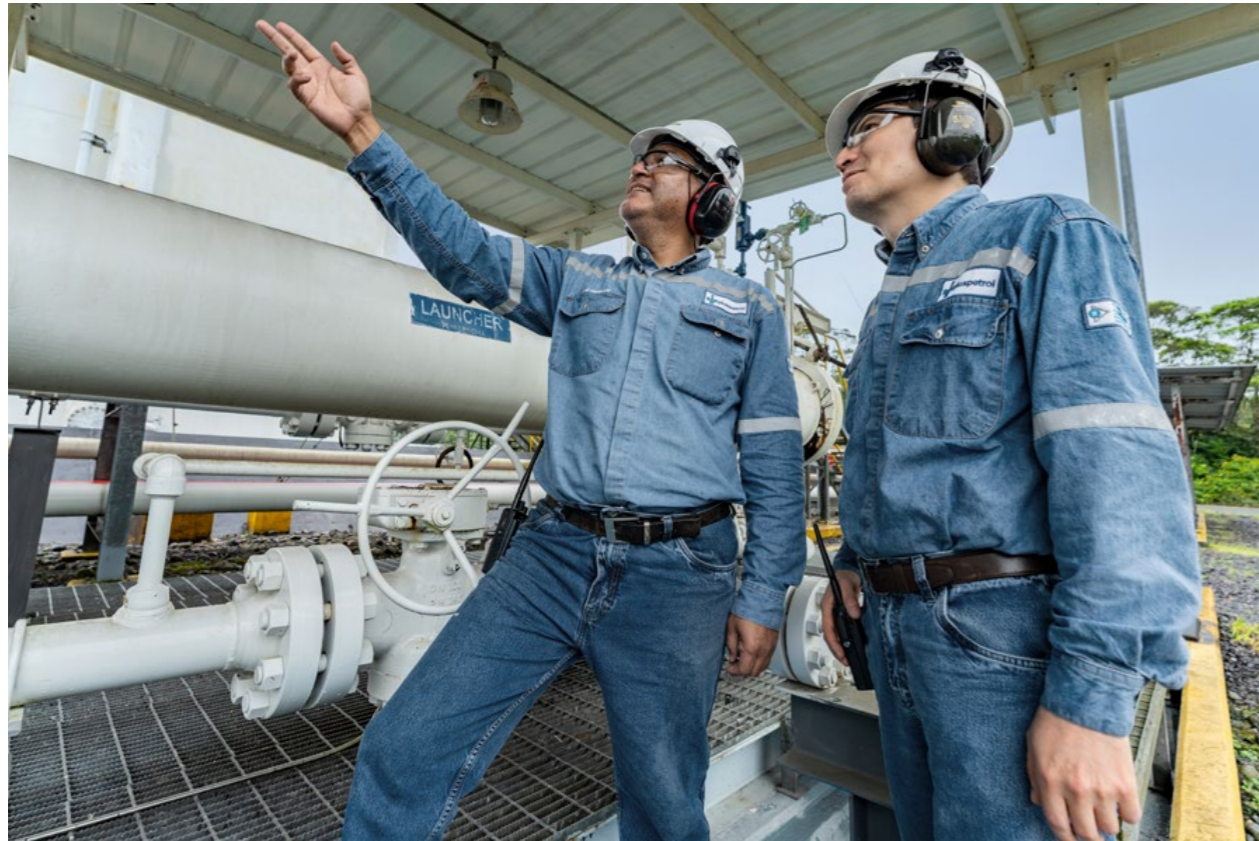
Central Processing Facility (CPF), Ecuador.
